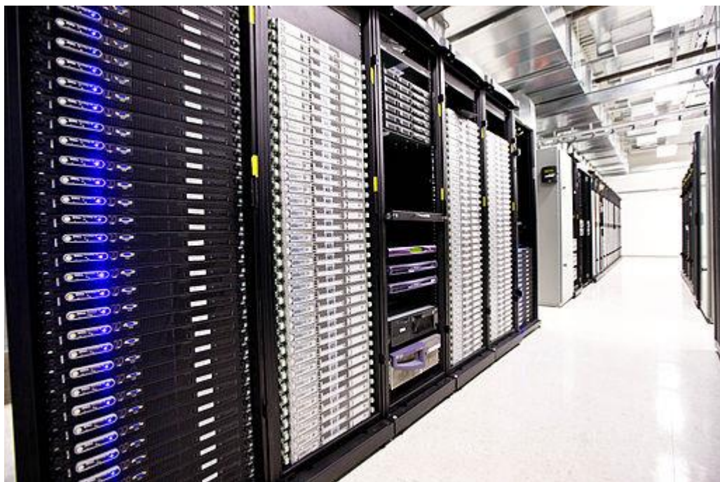
Figure 1 - Amazon Data Center
